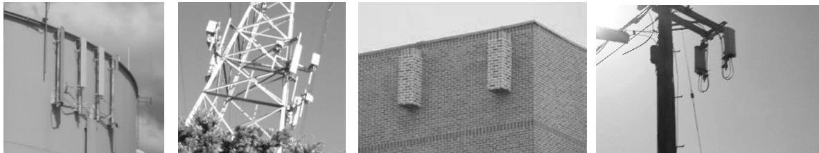
Examples of Flush Mounted Wireless Communication Facilities
