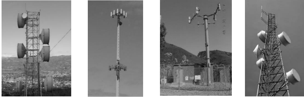
Examples of Non-Stealth Wireless Communication Facilities
