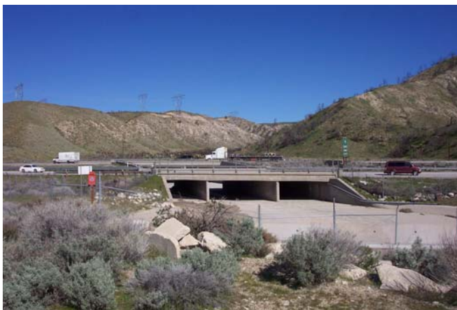
Figure 45. Gorman Creek undercrossing just south of I-5/SR-138 interchange, entering the State Water Project where it is funneled to Pyramid Lake.
