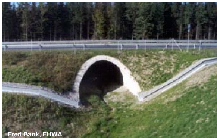
Figure 41. Arched culvert on German highway, with rail for amphibians and fence for larger animals.
