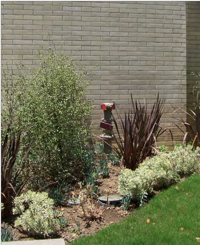
A back flow preventer that abuts the building and is screened from the view of the sidewalk and street by shrubs.
