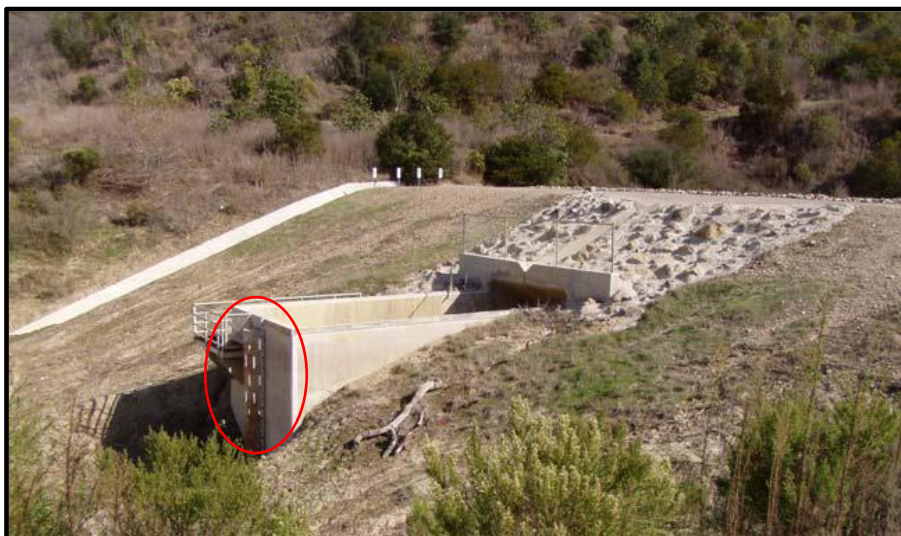
Figure 3-1 This debris basin includes a perforated “debris bleeder” made from a corrugated metal pipe (circled in red). (Source: VC Watershed Protection District)
