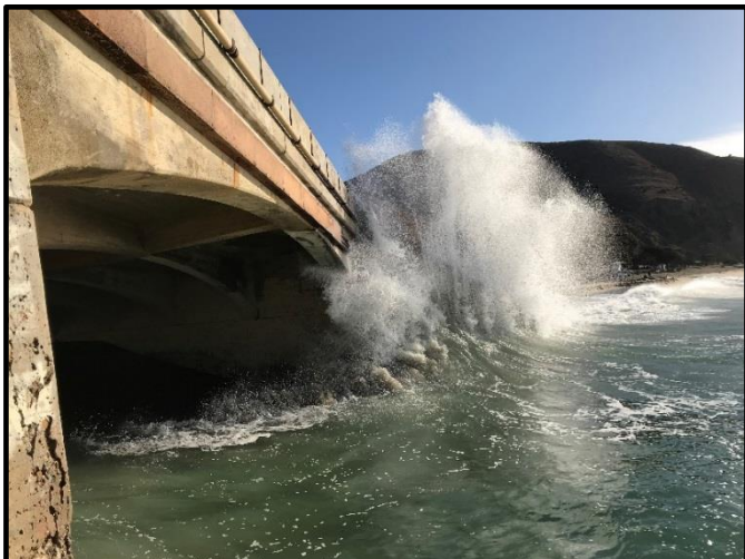
Photo 3-1: Sycamore Canyon Bridge located on the South Coast is 80+ years old and needs to be replaced. The new bridge will be built at a higher elevation.
