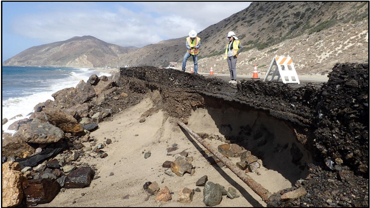
Photo 2-9. Erosion at Thornhill-Broome Beach that occurred on October 6, 2018 (Source: Caltrans).
