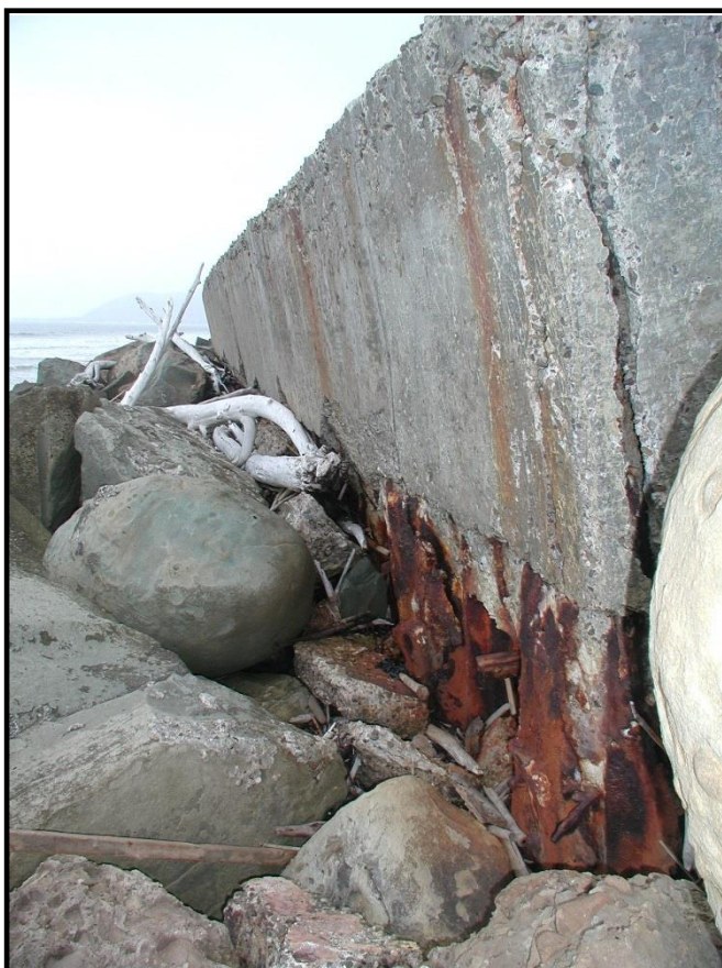
Photo B-2. Example of existing conditions of coastal armor along the Rincon Parkway.
