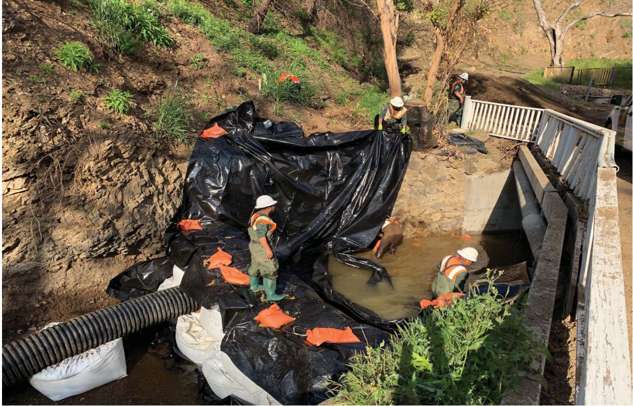
Photograph 7. Completing the temporary, upstream coffer dam of Diversion 1. Note visqueen around super sacks to avoid sedimentation within the creek (4/2/19).
