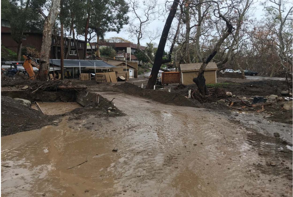
Photograph 1. View of fire debris on the pre-existing road and bridge (facing east) (2/15/19).
