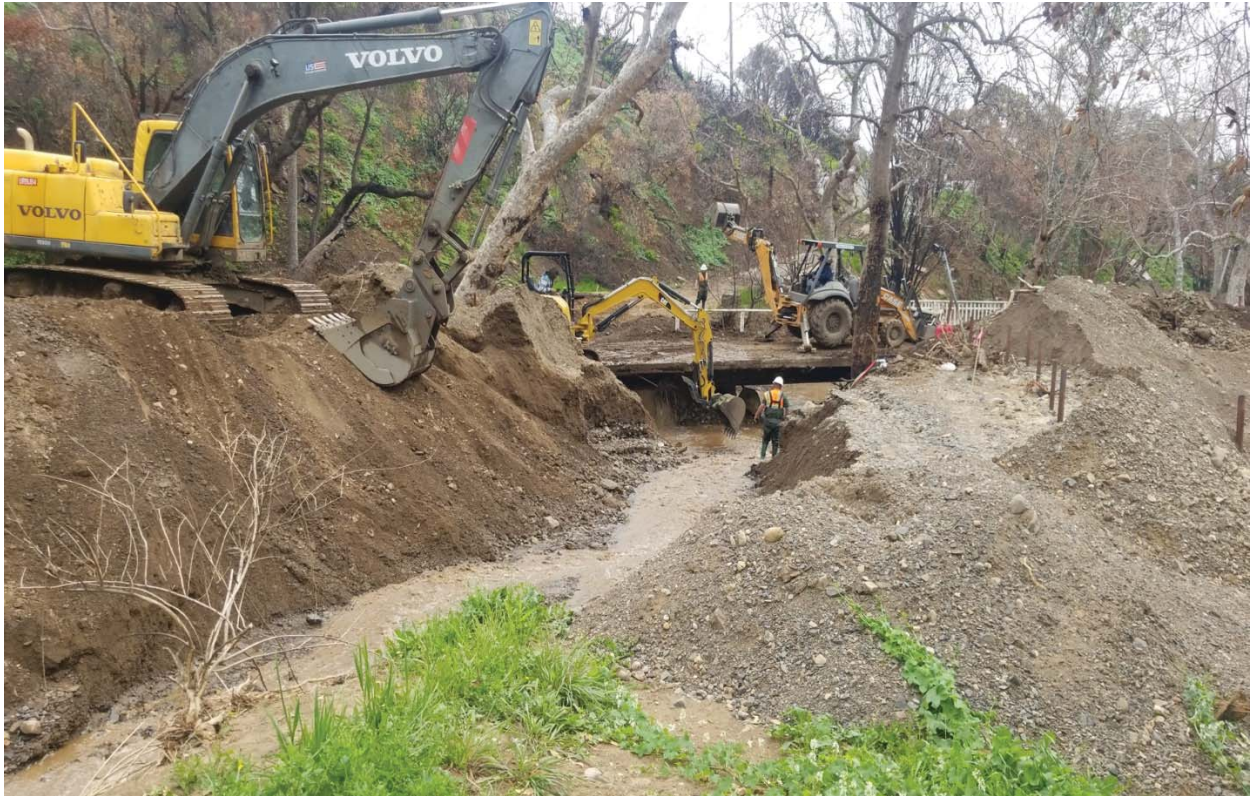
Photograph 3. View of equipment staged outside of the creek and removing sediment from the creek (facing south) (3/5/19).
