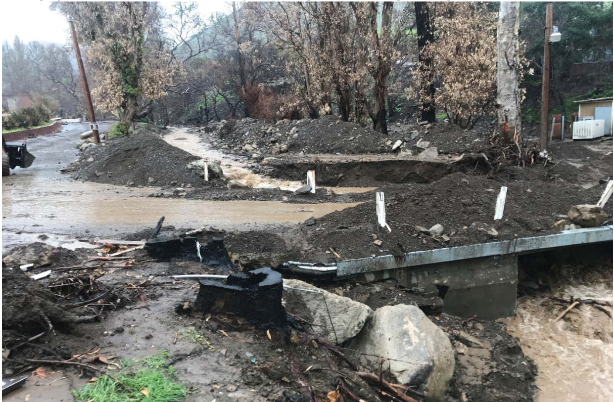
Photograph 2. View of pre-existing road and bridge, looking upstream within Little Sycamore Creek (facing north) (2/15/19).
