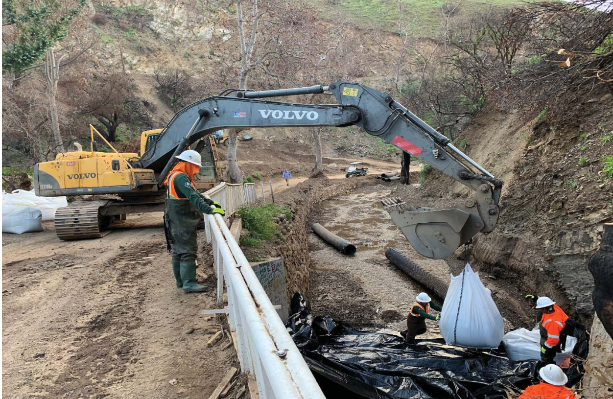
Photograph 5. Constructing Diversion 1. Note excavator lowering super sacks into the channel (facing south) (4/1/19)
