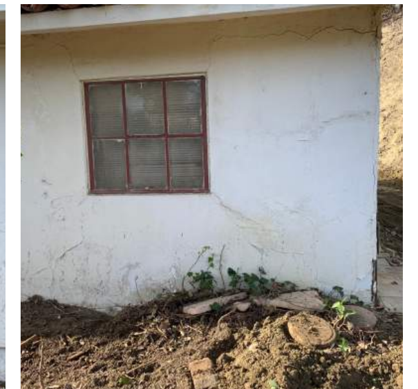
Building H2 Exterior Damage Billiwhack Ranch
