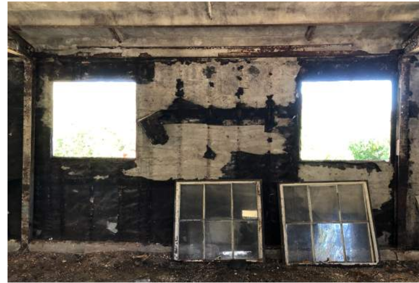
Studs and water membrane gone
