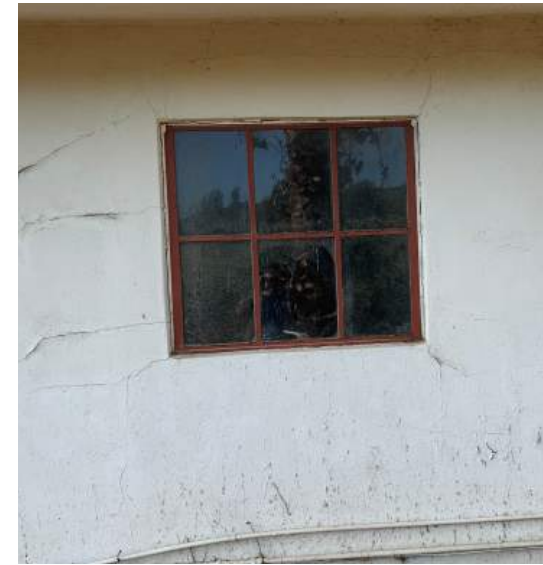
South Side: Stress fractures & damage visible at each window
