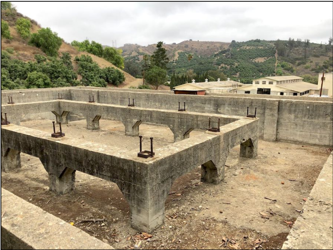
Photo 18. Hammer Mill, view from southwest. [9-27-19]
